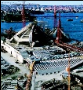
The Podium takes shape at Bennelong Point. Photograph by Max Dupain and Associates
